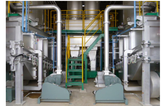
Biomass boiler at Odate Plant
